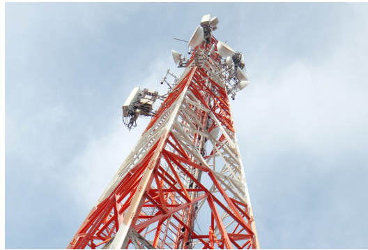
Self-support tower (SST): Tower with height of 30-72m with 4 or 3 legs
