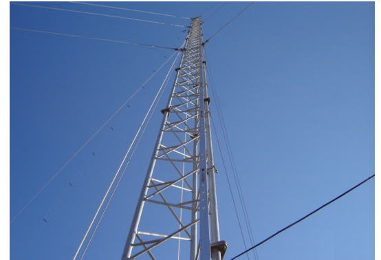
Guyed mast: Tower with only a single pile and supported by steel
