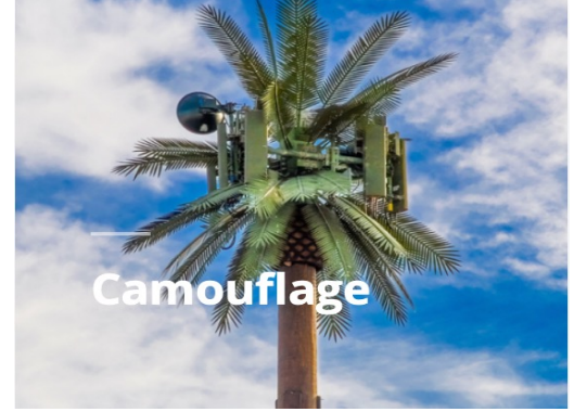
Camouflage: Smart pole used as public lighting, CCTV, digital signate, integrated broadband and IoT connectivity
